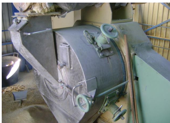
Figure 5 - The granulator of the working installation
