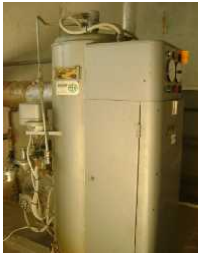
Figure 1: The steam boiler type Certuss Junior used in the processing installation
