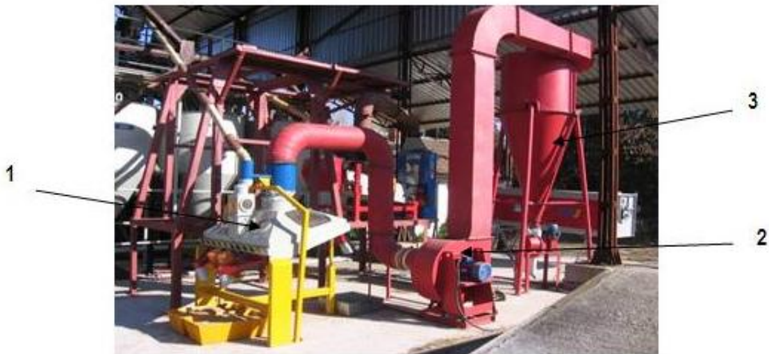
Fig.3. General view of the installation used in experimental research
