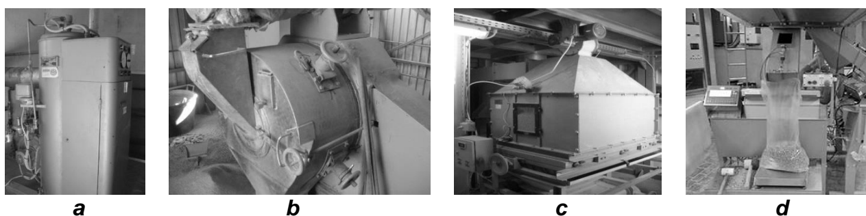
Figure 4 - Working installations from a compound feed factory: steam generator (a), granulator (b), cooling plant (c), packing plant (d)
